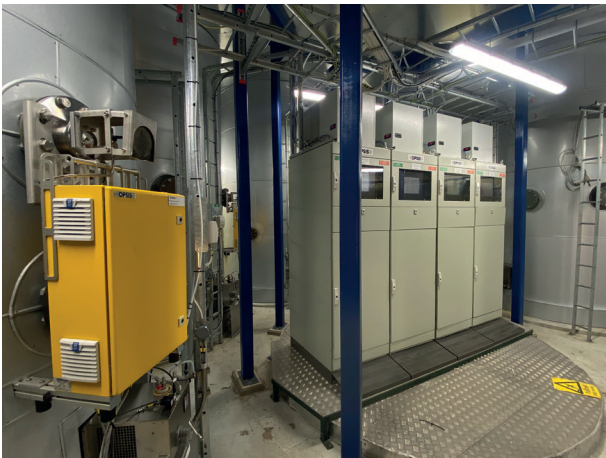
Fig 1 Photo shows one of four stack-mounted OPSIS automatic dioxin sampling boxes (yellow box) and four DX100 control cabinets at a large Swedish waste-to-energy plant.
