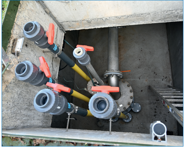
© WMD, Hydrostatic level measurement with a KELLER data logger
