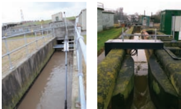
Fig 1: Feed Forward Control involves taking a sample at the inlet prior to the addition of chemicals.
