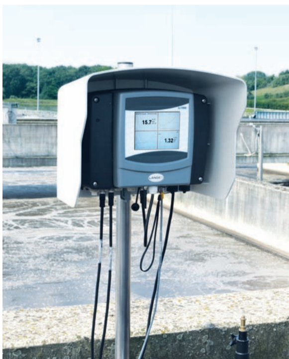
Figure 2: SC1000 Controller at an aeration tank
