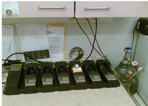
Figure 5: Automated calibration equipment
