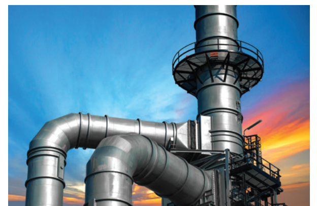
Power plant stack emissions
