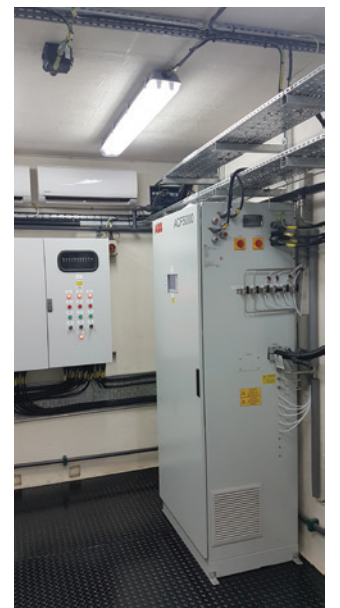
Copyright ABB - ACF5000 FTIR CEMS installation
